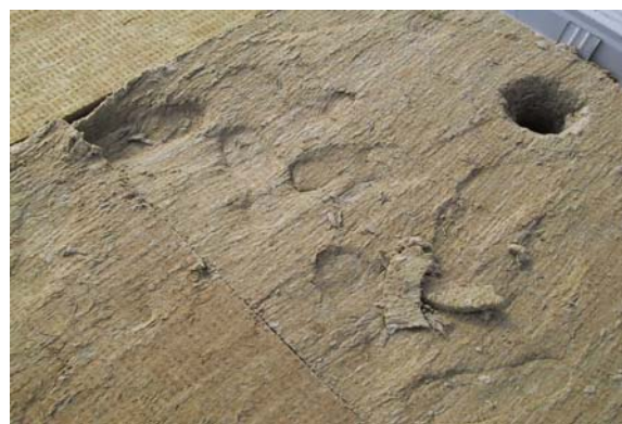
Fig. 1. Insulation board (in dimensions 1200 mm × 600 mm) destructed by pedestrian traffic
