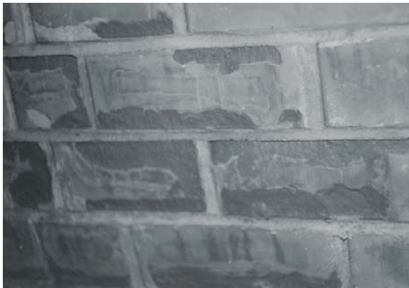
Fig. 3. The fragment of ceramic finish brick masonry impregnated with a hydrophobic material after testing by simulated effect cycles in the climatic chamber
