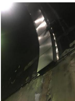
Fig. 1. Water box at a leak in the lining
