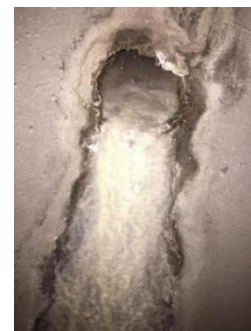
Fig. 3. Crystal blockage of a drainage pipe
