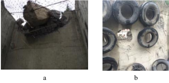
Fig. 1. Disaster caused by rockfall: a—RC-slab damage cases; b—retaining wall damage cases
